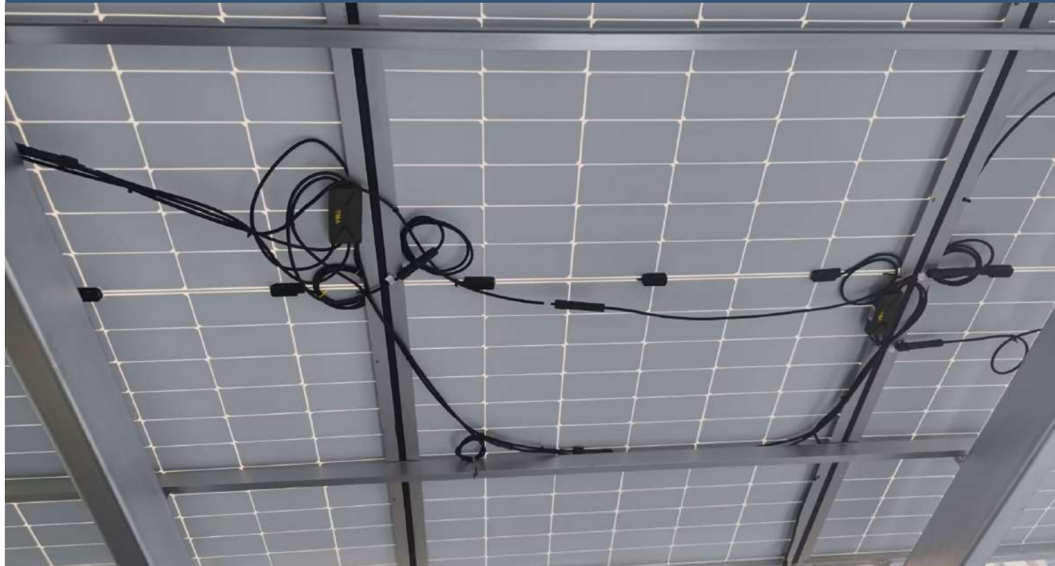
33 kW Solar Parking in Bangkok, Thailand
